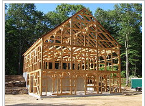
The skeleton of a post and beam horse barn just after raising
