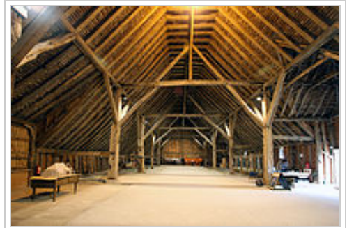
Grange Barn, Coggeshall, Colchester, England, originally part of the Cistercian monastery of Coggeshall. Dendrochronologically dated from 1237–1269, it was restored in the 1980s by the Coggeshall Grange Barn Trust, Braintree District Council and Essex County Council.
